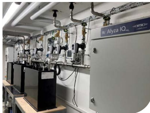
Fig. 3, top: The graywater recycling room with 2-stage biological treatment and UF of the graywater
